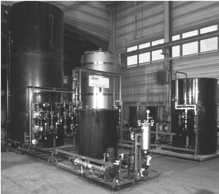
Fig. 9.12 Calmix® plant (Source: EUWA).
