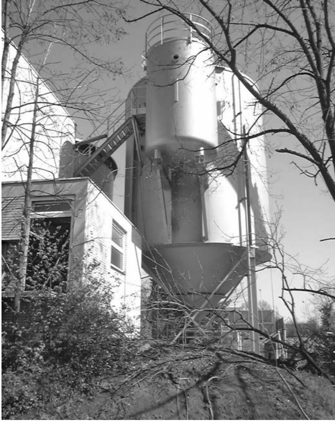
Fig. 9.6 Lime softening plant (Source: EUWA).
