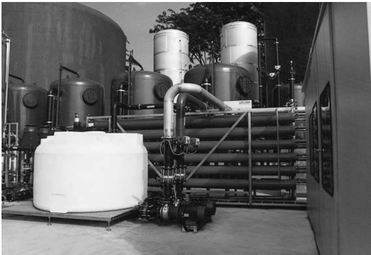
Fig. 9.10 Reverse osmosis plant (Source: EUWA).
