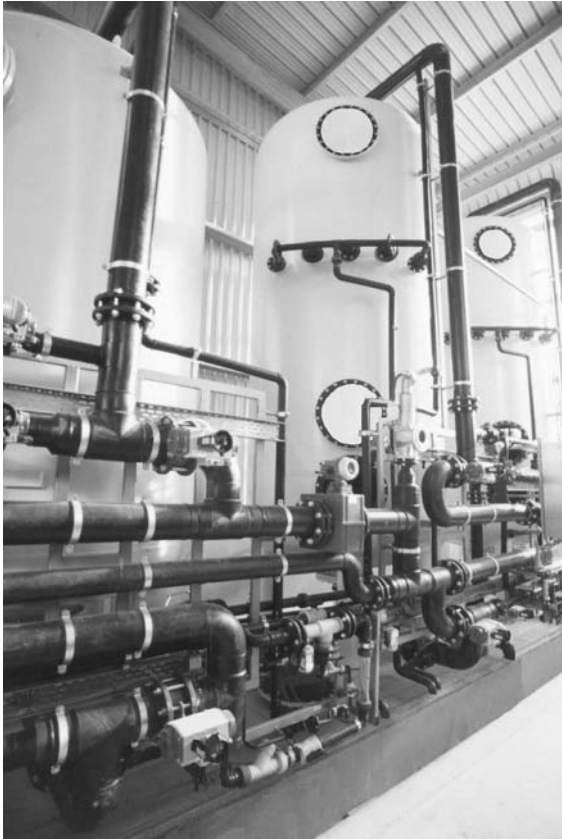
Fig. 9.8 Ion exchange plant (Source: EUWA).
