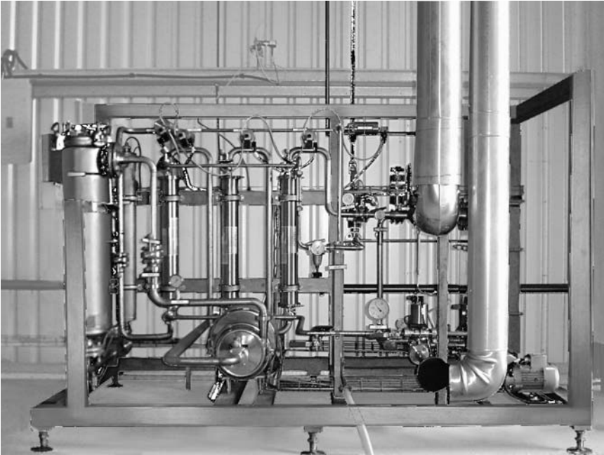
Fig. 9.14 Erox deaeration plant (Source: EUWA).
