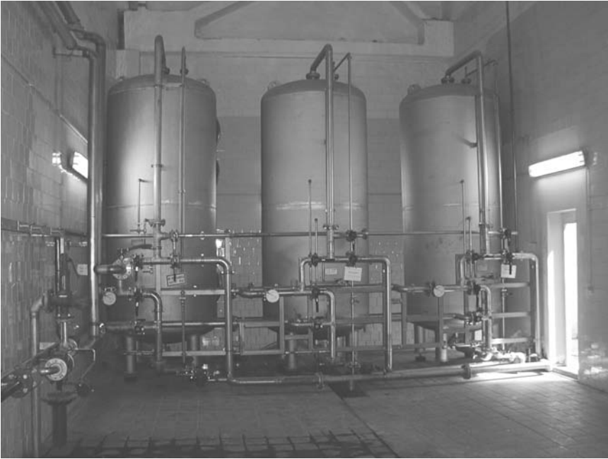
Fig. 9.4 Activated carbon filter plant (Source: EUWA).
